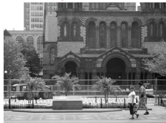
The City of Boston has begun work to renew the lawn and some of the masonry in Copley Square. See page 3 for details.
